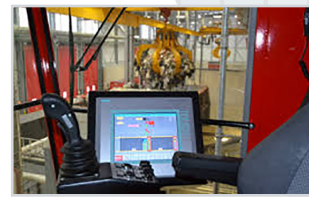
HMI Operator Display Panels
